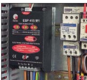
ESP 415 M1 installed within a control panel on the mains input to protect the panel's control systems. Note the remote indication connection (top of protector)
