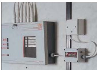
Ready boxed protector (here an ESP 240-5A/BX) installed on the fused connection (spur) to an alarm panel
