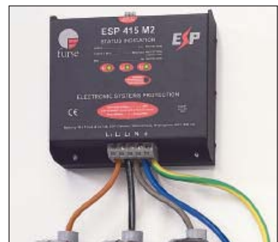
Live connecting leads should be fused accordingly
