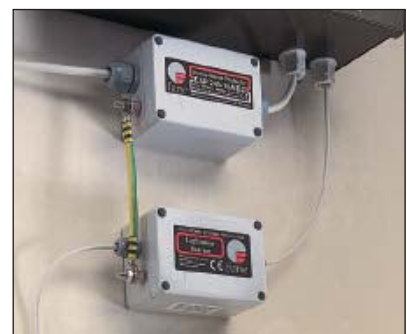
Security alarm panel with ESP TN/BX (bottom) providing protection from transient overvoltages on the dial-up telephone line. Note how the ESP TN/BX is earthed via a bond to the ESP 240-16A/BX (top) installed on the mains power supply to the panel
